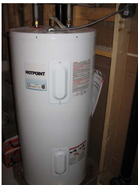
Figure 7: Hot water tanks often come preset at 60 °C. To keep the water at this temperature, the tank uses more electricity than it would if the temperature was set a five or ten degrees lower. While the savings would be huge, the amount of hot water available to the household would not be reduced.
